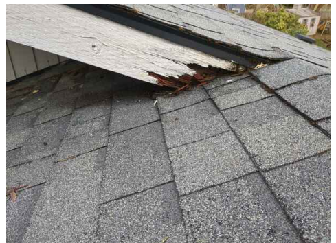
this is above the front entry way where the fascia meets the peak of the garage
