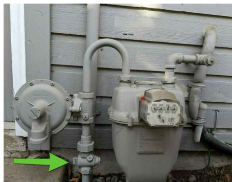
natural gas shut-off
