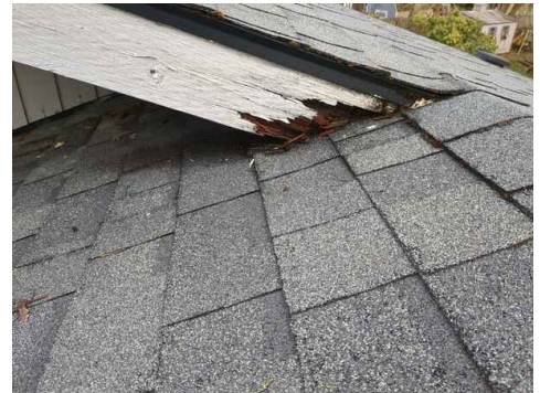
this is above the front entry way where the fascia meets the peak of the garage roof.
